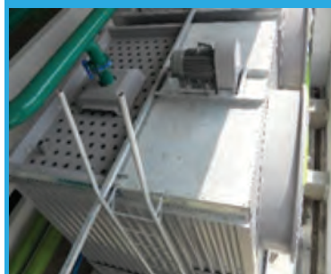
Hot Water Basin
